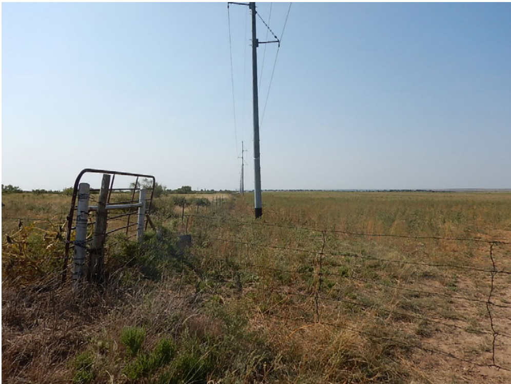
Photo 4. Typical view of existing overhead transmission line ROW within Route Option B, facing south.
