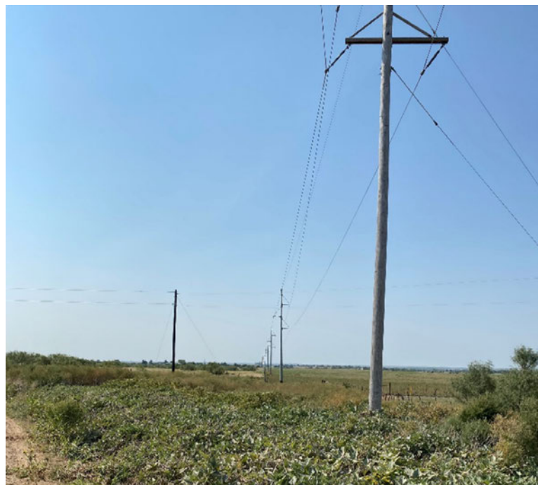
Figure 15 – Existing Electric Transmission Line Along County Road I, Facing South
