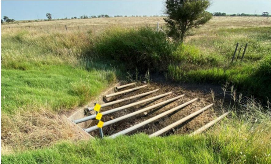
Figure 10 – Typical Drainage Outlet Along SH 70
