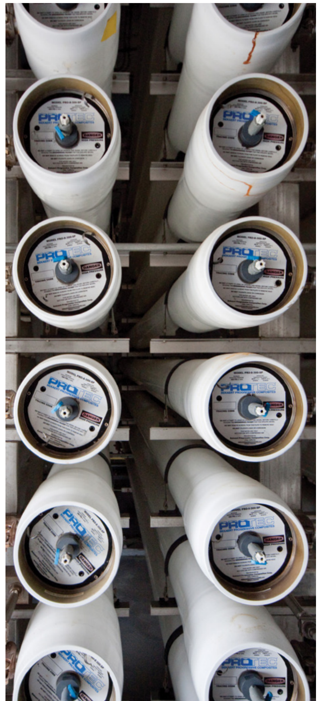
Reverse osmosis membranes at a brackish groundwater desalination plant
