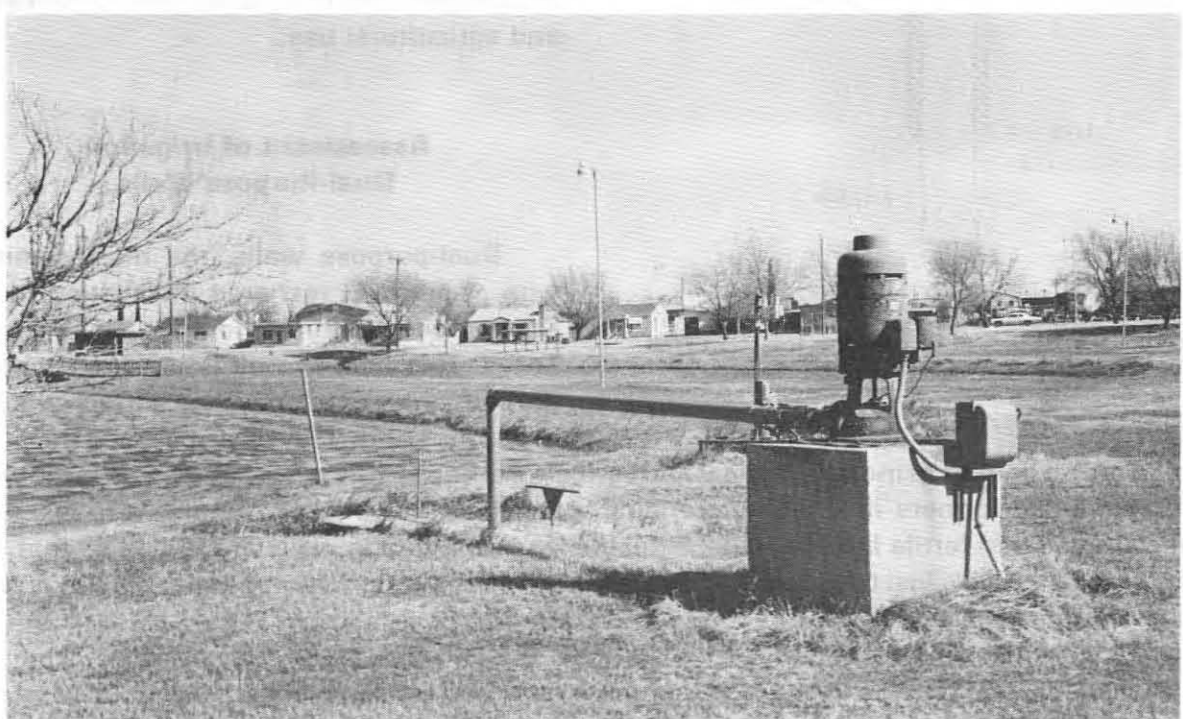
Figure 8-8.—Recharge Well for Playa Water in Lamesa, Dawson County
