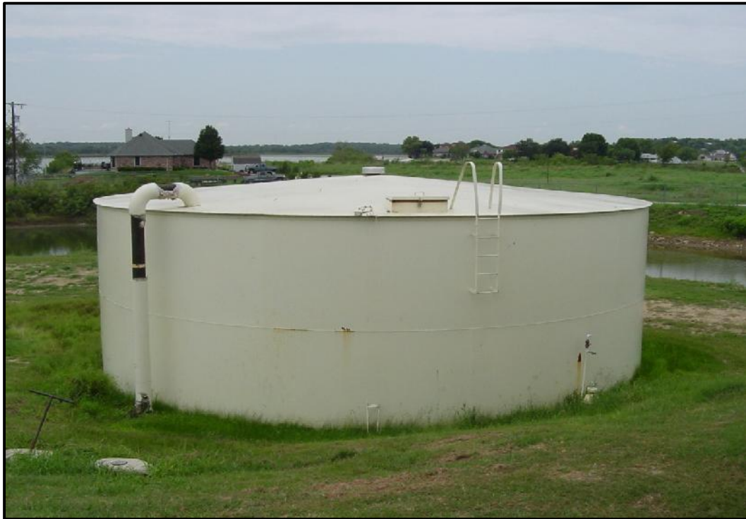
100,000 gallons storage tank
