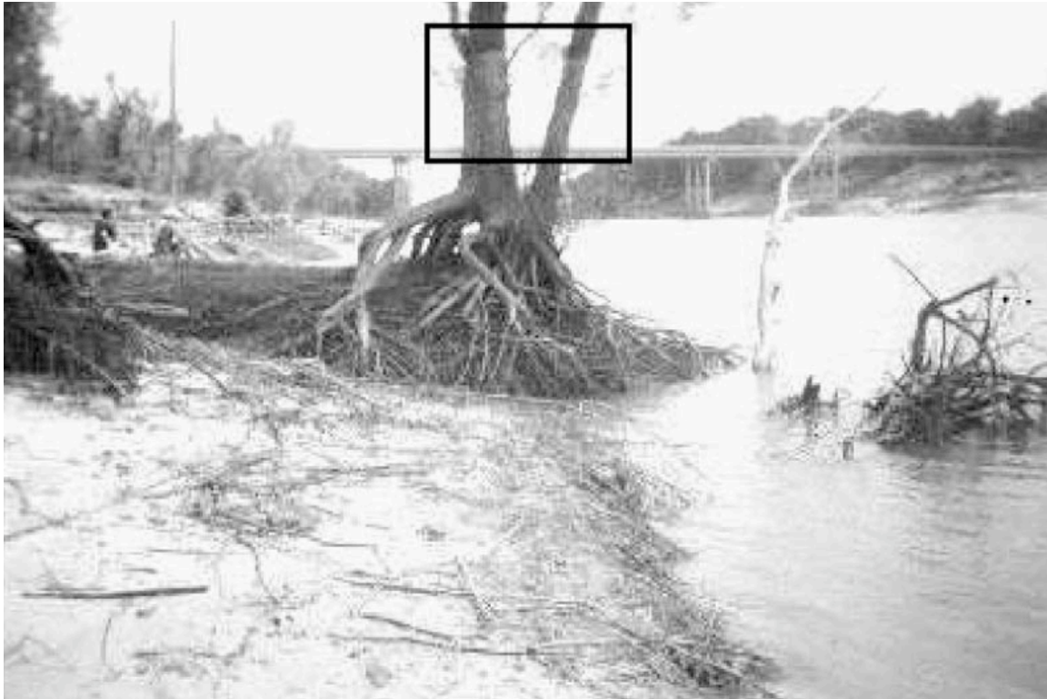
Figure 11. Scour zone below Livingston Dam on the Trinity River. Exposed tree roots indicate downcutting and bank retreat. The gray stains on the tree trunk (box) are due to scour of the clayey bed material beneath the thin alluvial layer.
