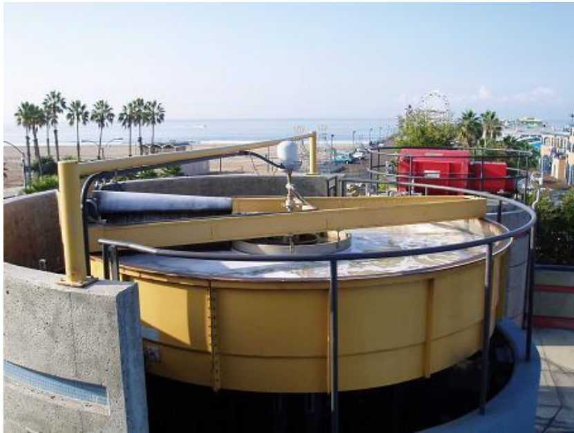
Figure 8-2: Dissolved Air Flotation Treatment at the SMURRF
