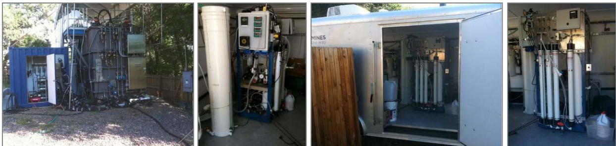
Figure 4.19 The pilot forward osmosis/reverse osmosis system deployed at CSM Wastewater Research Facility
