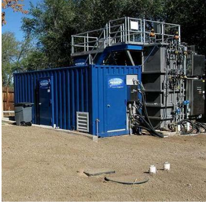
Figure 4.17 The SBMBR demonstration system at CSM (Golden, CO)
