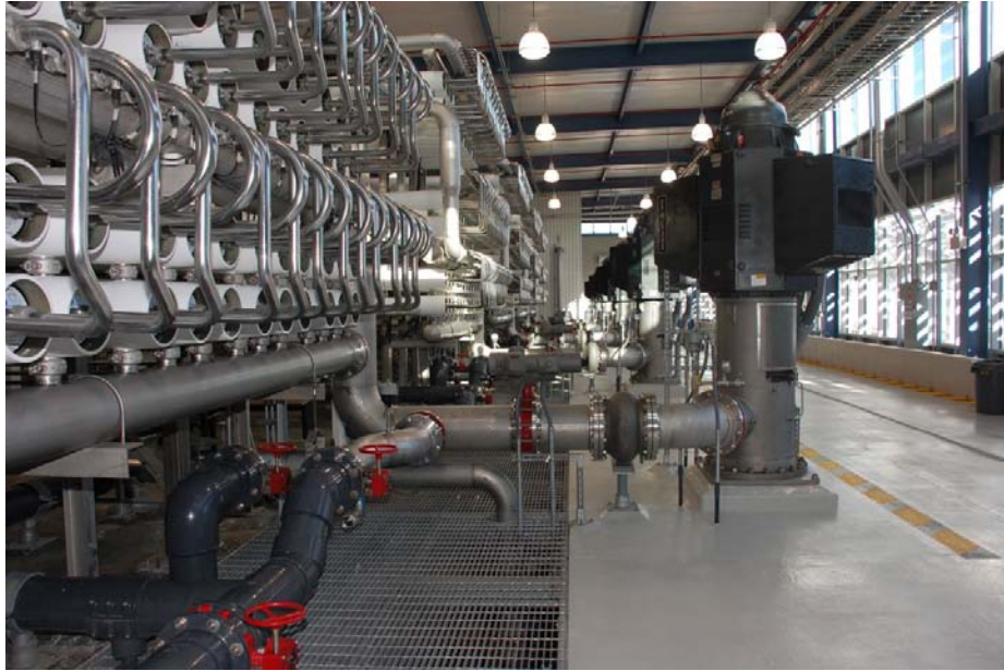
Figure 2.6 Kay Bailey Hutchison Desalination Plant, El Paso (Photo credit – El Paso Water Utilities)
