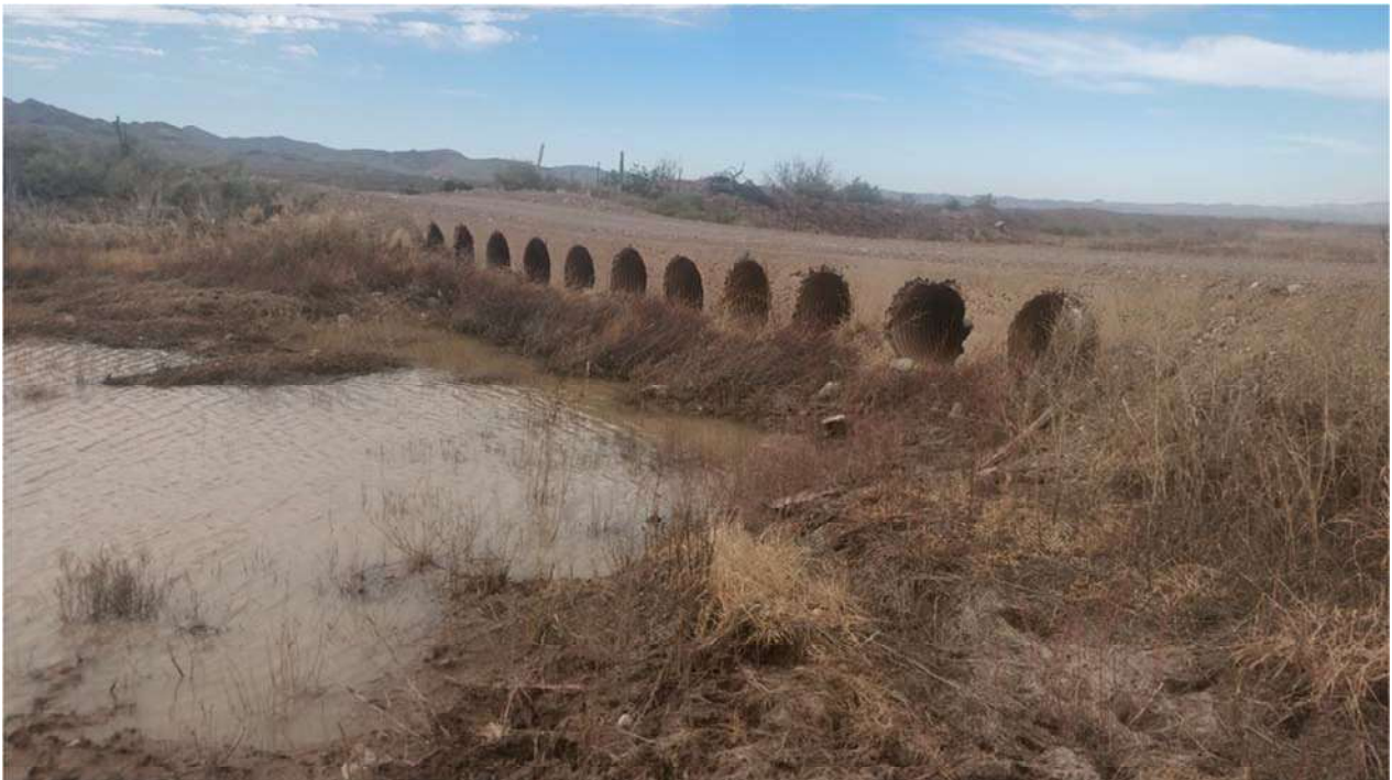
Figure 1: Wild Horse Draw – Eleven 36" Diameter CMP Culverts
