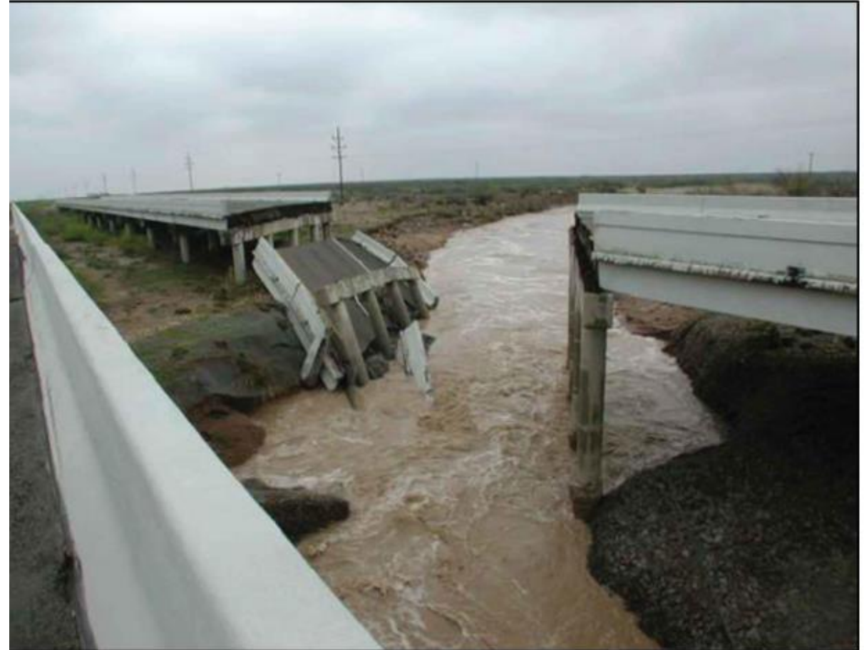
April 2004 flood caused this I-20 bridge over Salt Draw to collapse, located between Toyah and Pecos. Source: DAA and NWS; https://www.weather.gov/maf/2004_04_02_SevereWeather
