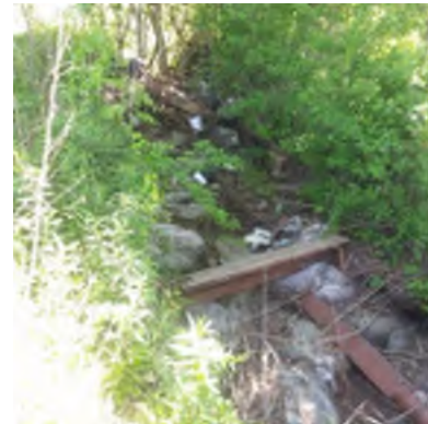
Figure 2-3: Illegal Waste Disposal on P118-25-01
