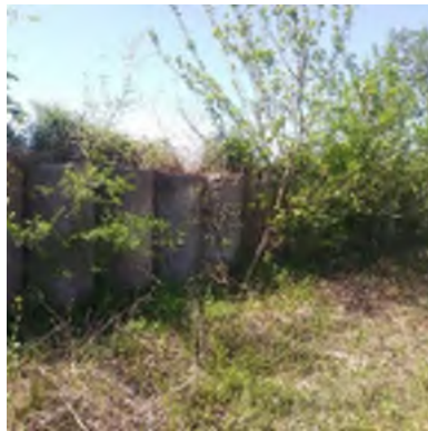
Figure 2-2: Misuse of Culverts on P118-25-01 South of Henry Rd
